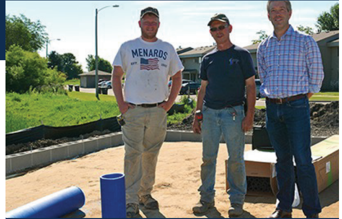
Left to right: Maury Erickson, master installer for Chappell Central; Dylan Olson journeyman installer for Chappell Central; Kevin Herrema, sales engineer for SVL
