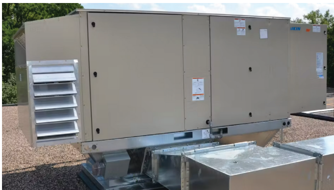
One of Bethel's new Daikin Rebel rooftop units
