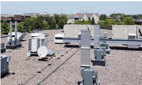
Photo: Be The Match® Rooftop Units
